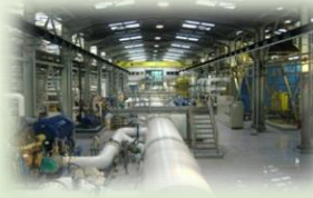
Skikda (Algeria) 100,000 m 3 /ay
